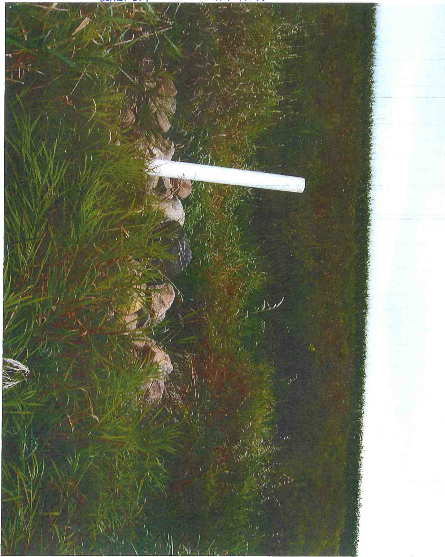
WASH-OUT FILLED WITH ROCK
