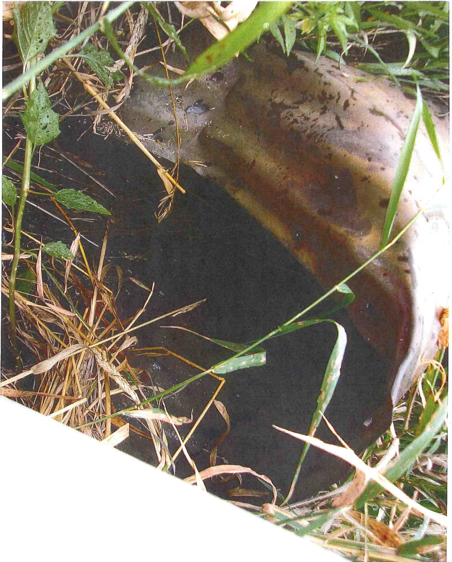
END OF EXISTING Gmp BENT, RESTRICTING FLOW
